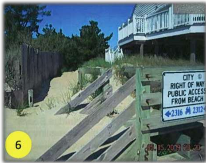
Figure 8. Sand dunes overtaking wooden structures.
